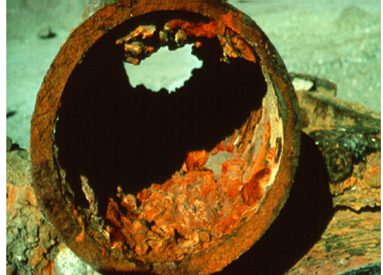
Salinity damages to municipal water pipe.
