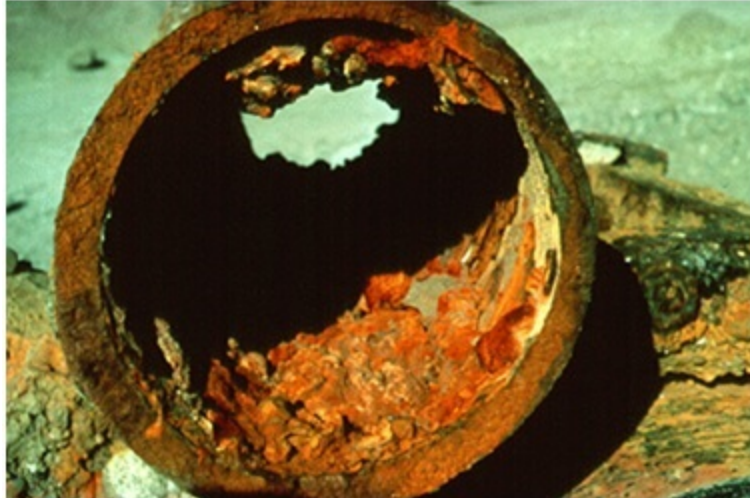
Figure 2. Salinity damages to municipal water pipe
